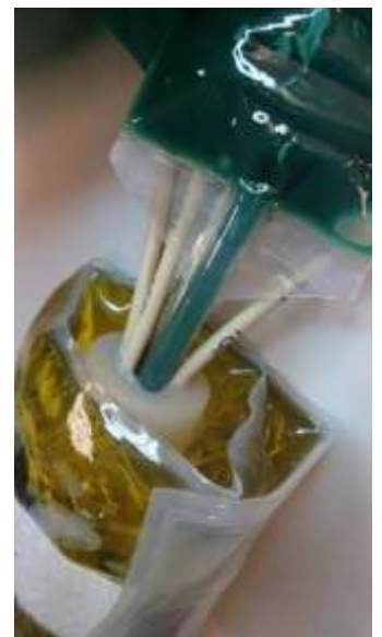
Figure 3 - RapidEx installation with Industrial Gland Warmer in position
